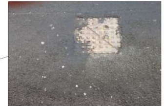
Evidence of sewer crossing through Swine Market - chamber lid in Cow Green
